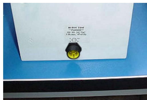
Figure 5 - DC Power Connection
